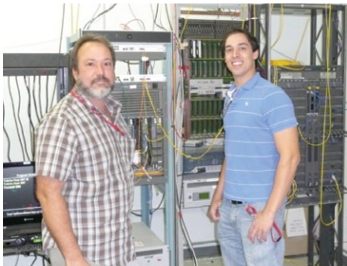
Jim Bortolini, Communications Engineer and Ben Rose, Engineering Technician, perform testing on the communications system.
